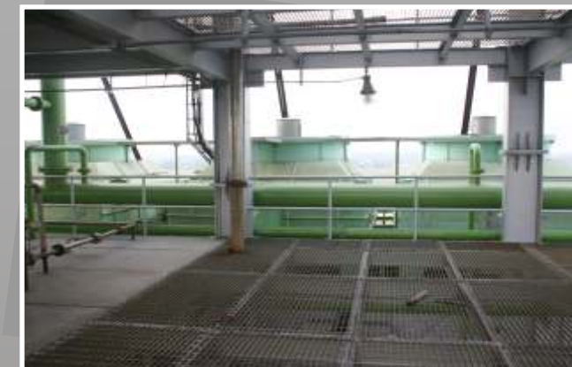
Cooling Tower & Pipe Line
