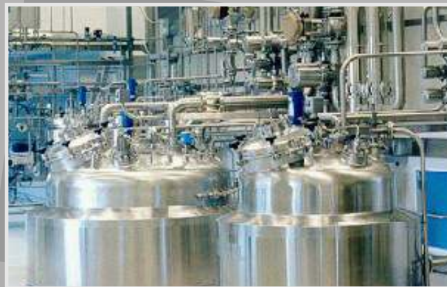
Medicine Plant Reactors
