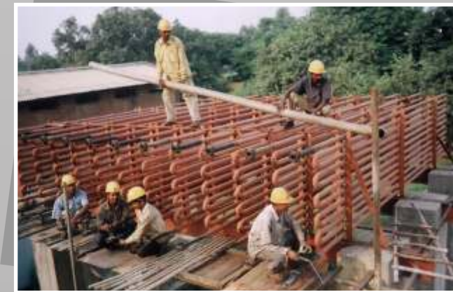
Chilling Plant Open Condenser
