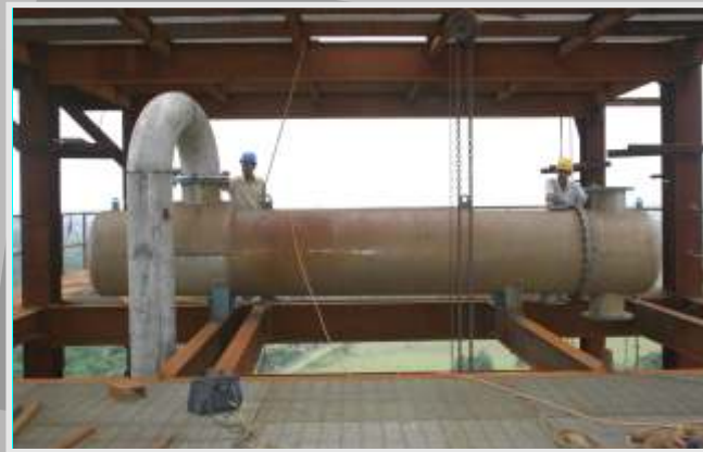
Distillations Main Heat Exchanger
