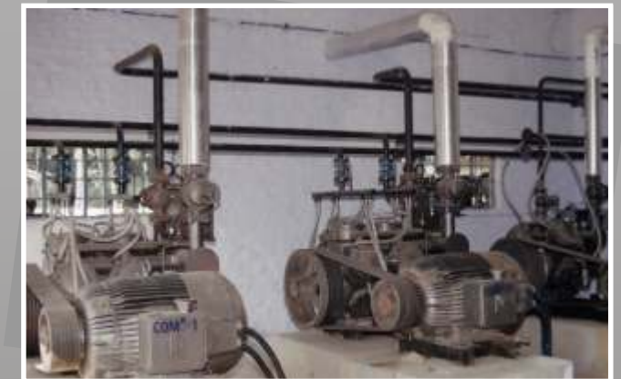
Chilling & Brine Compressor
